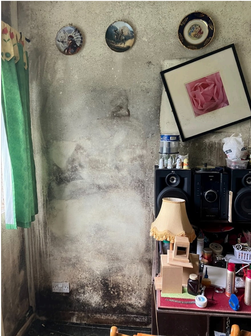
Black mould in the house of a disabled Thirteen tenant in Billingham
